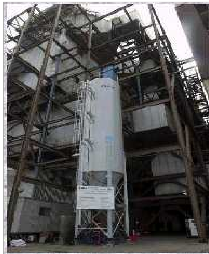
Activated carbon storage and feed system
