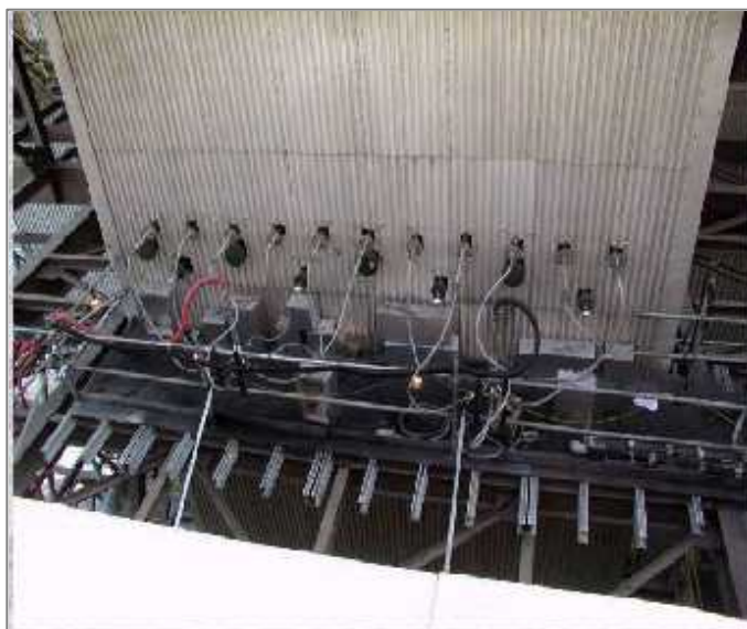
Activated carbon injection system
